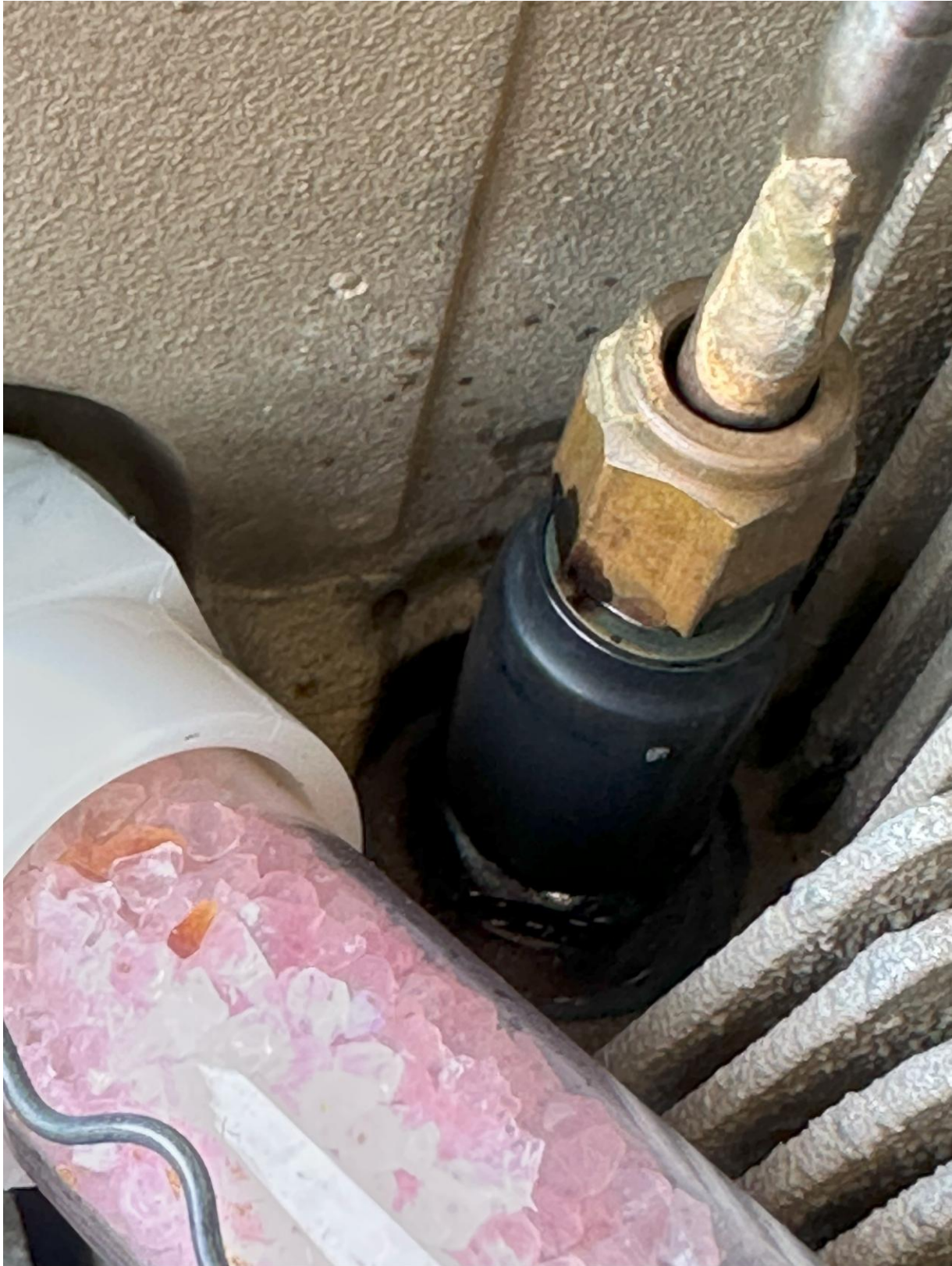
Here is some black coating on the outside of my fuel injector taken during annual. My mechanic says this coating is not found when 100LL is burned.
